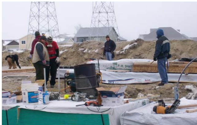
Through the cold Montana winter, families and volunteers worked to make the dream of homeownership a reality.
